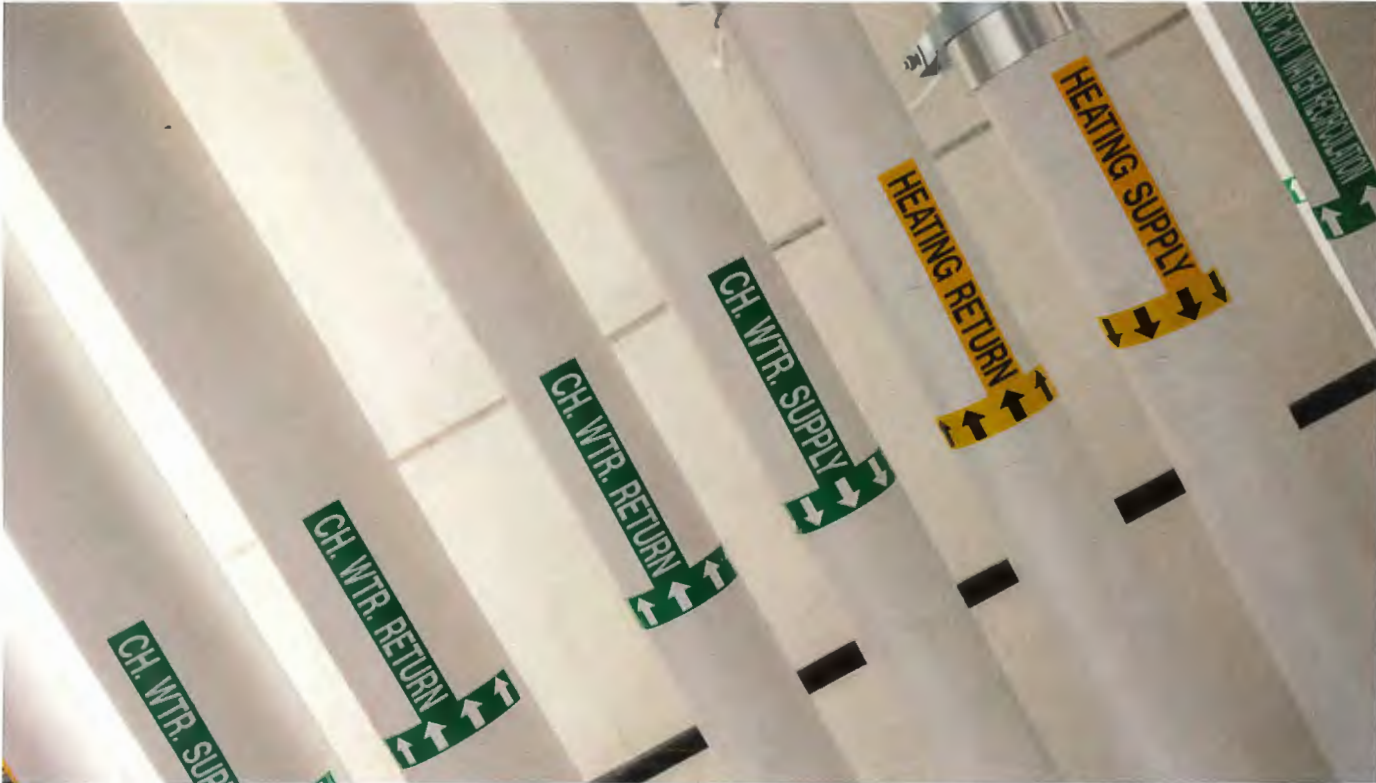
Interior supply and return piping located at the recently connected One Park.
