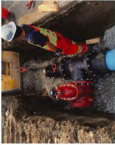
Staff helping an excavator line up a fitting during a watermain capital construction project.
