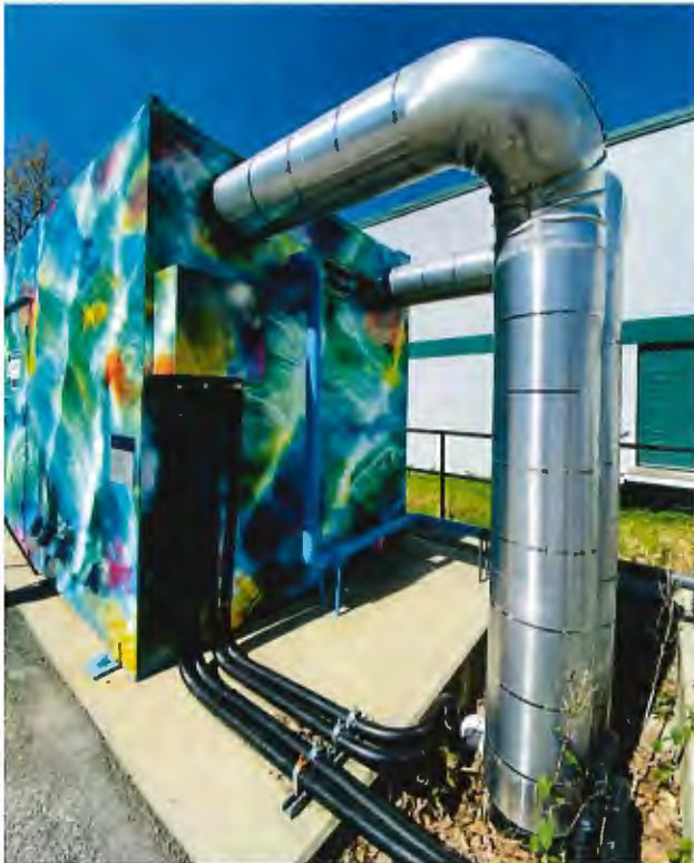
Oval Village District Energy Utility
