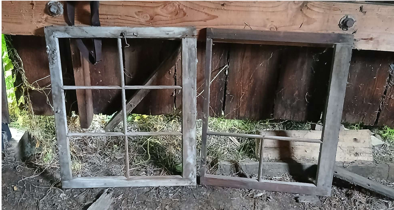
May 2026 photograph of two wood sash, remnants in room 1, currently sitting on the ground however they come from openings located in this room.
