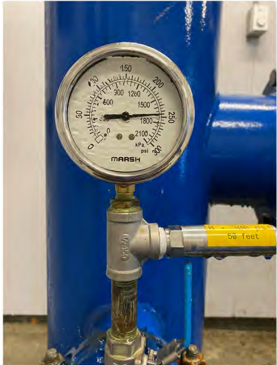
Metro Vancouver water connection to PRV station
