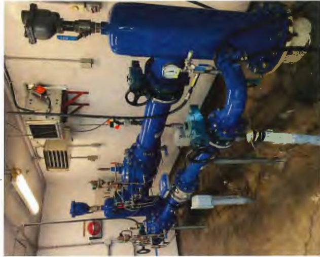
A look inside a pressure-reducing valve station.
