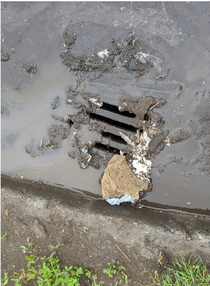
Solids and litter clogging a catch basin on Mitchell Island.
