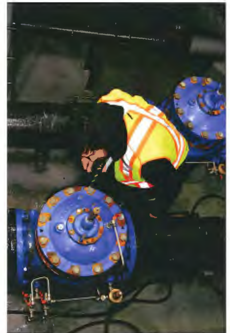
Inside a PRV station
