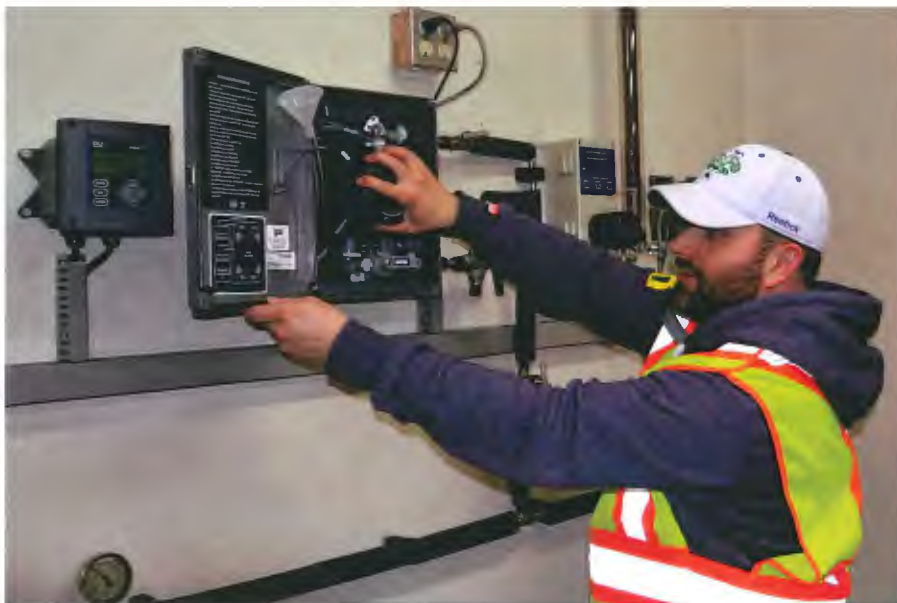
Inside a PRV station
