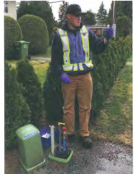
Taking a sample of the chlorine residual
