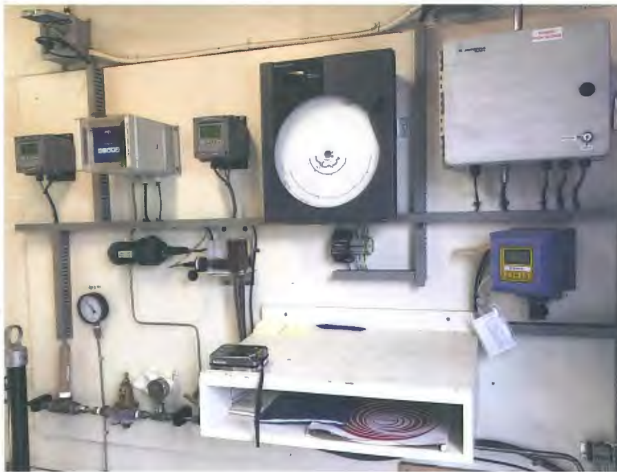
Data acquisition inside the PRV
