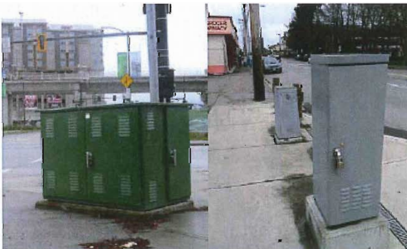
Figure 3. Examples of existing utility boxes in Richmond.
