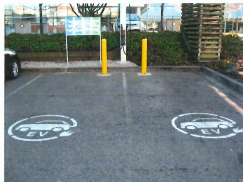
Figure 5: EV Charging Station at City Hall
