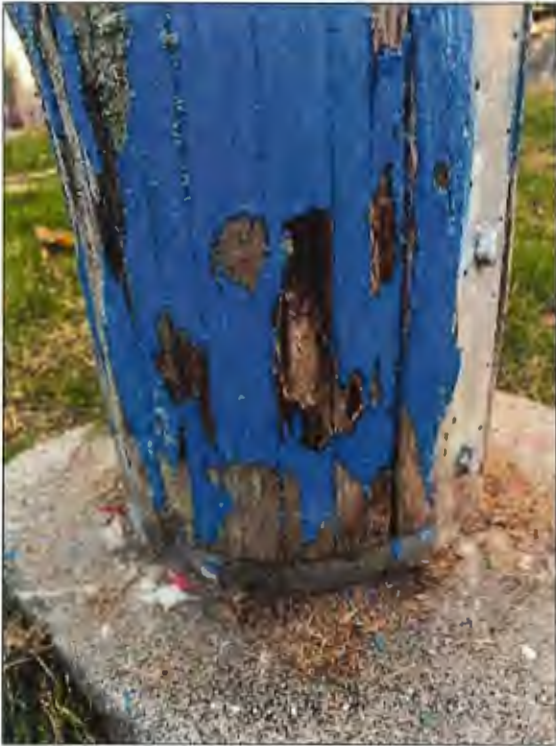
Insect damage, paint loss and wood rot
