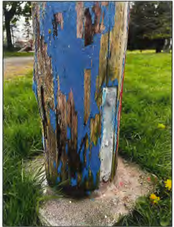
Insect damage, paint loss, and wood rot
