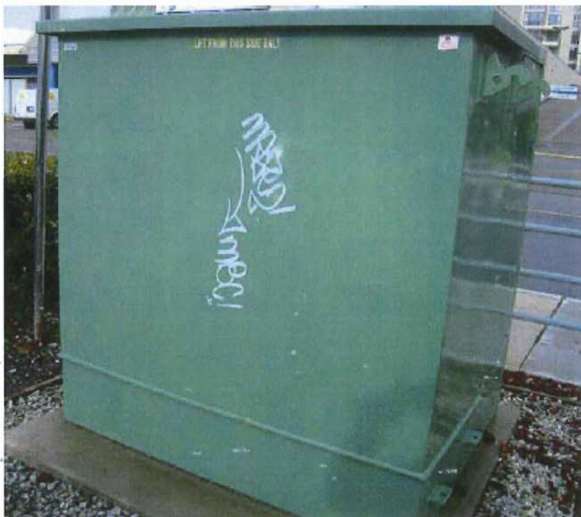
Figure 1. Example utility box tagged with graffiti.
