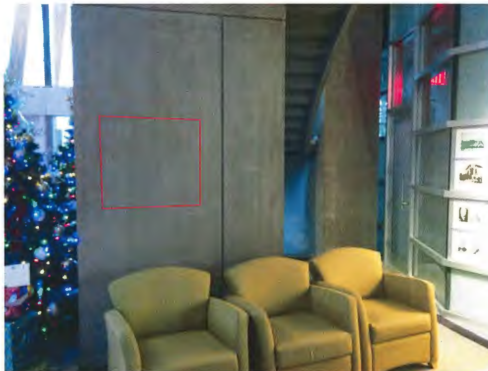
Figure 2.1 (top) and 2.2(bottom) – Proposed location on concrete pillar at public seating area, outside Council Chambers.
