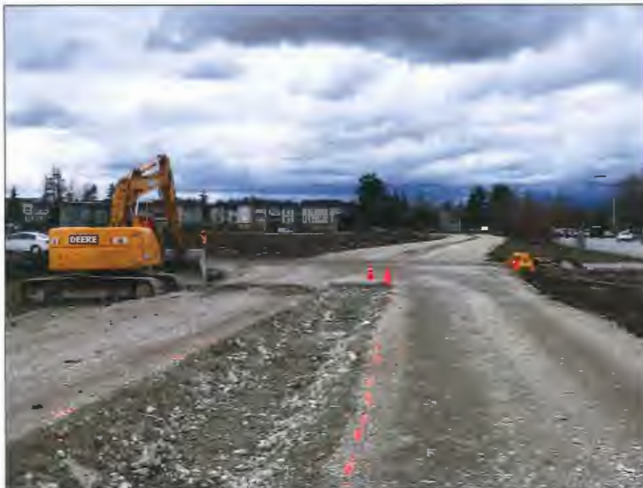
Above: Substantially complete portion of bicycle and pedestrian paths along No. 4 Road. Final top layer of fine gravel not yet installed.
