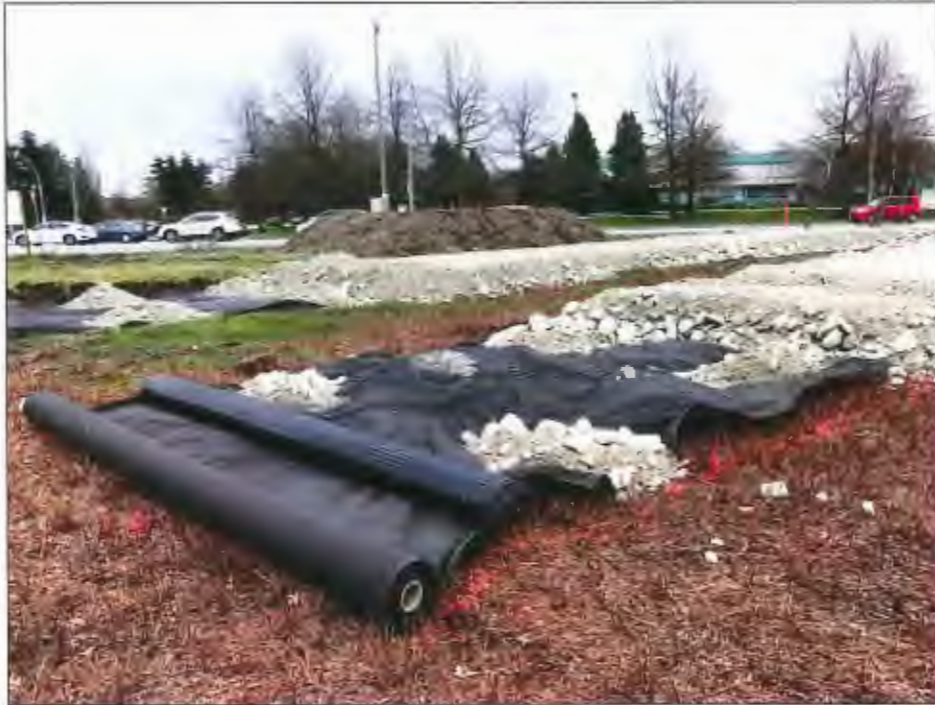
Above: Initial stages of perimeter path construction (geotextiles and crushed stone base layer) along No. 4 Road.
