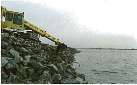
City crews continually maintain and upgrade the City's diking infrastructure. The Dike Master Plans Phases 1 to 5, anticipated for completion in 2019, specify upgrade requirements for Richmond's dikes according to current climate change science.
