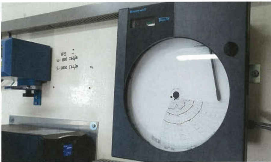
Data acquisition inside the PRV
