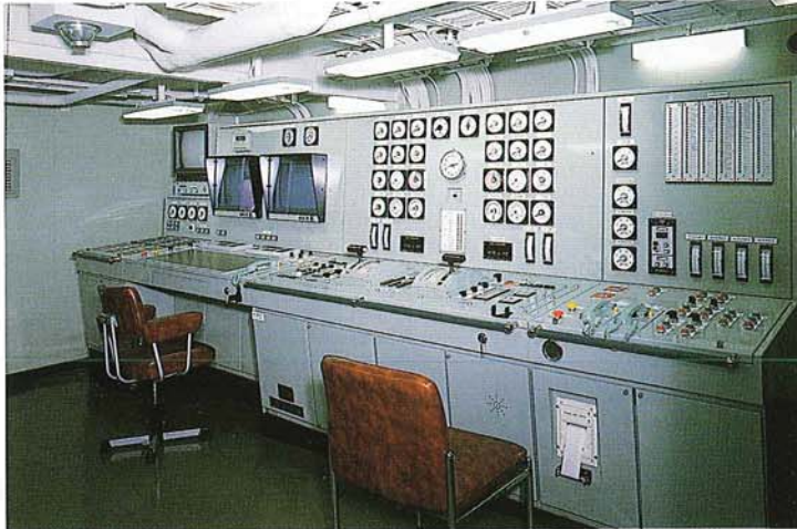
Engine control room
