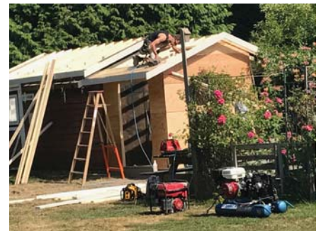
The Bee House and Shed were refurbished and rebuilt to provide dry storage and safe housing for the bee hives.
