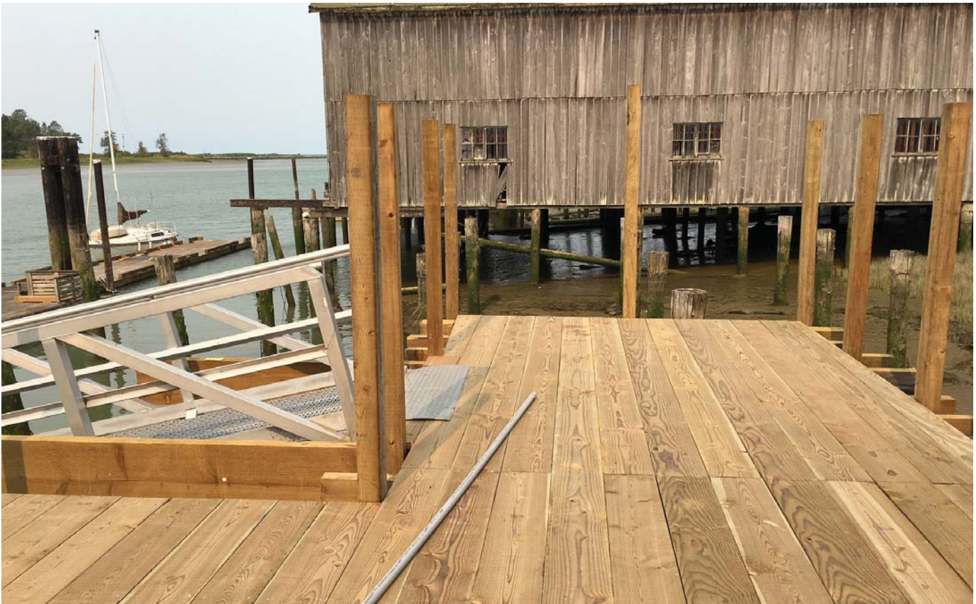
The new Seine Net Loft walkway and decking was installed in the summer of 2017.
