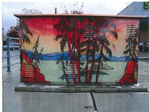
Ackroyd Pump Station
