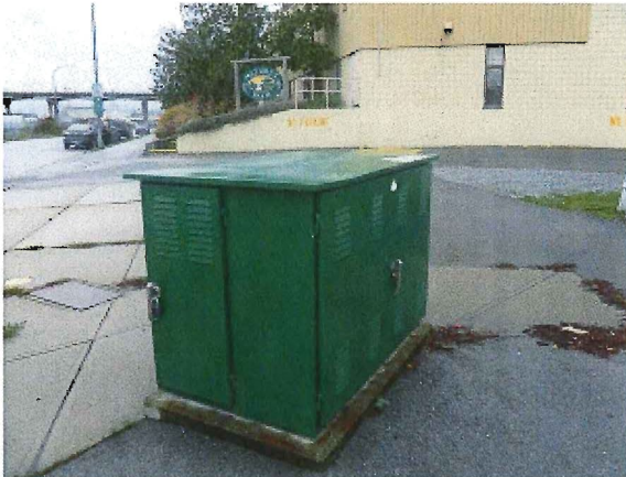
Van Horne Pump Station (9031 Bridgeport Rd.)
