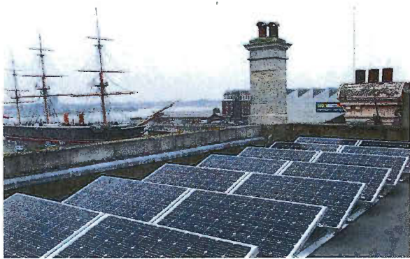
Solar panels behind a false parapet on a flat roof
