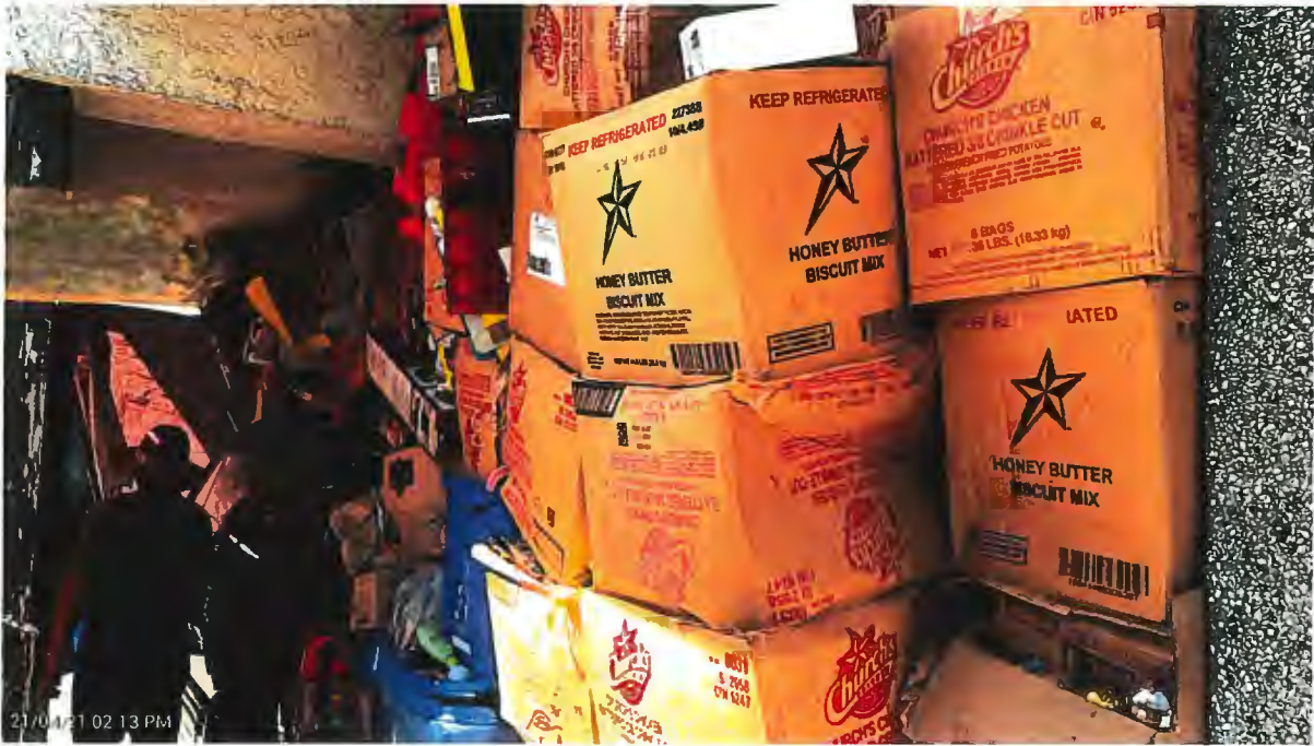
Carport is full of boxes of newspapers and books and two derelict vehicles. 10100 Severn Drive – Photos taken April 21, 2021
