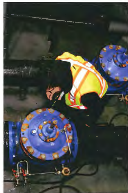
Inside a PRV station
