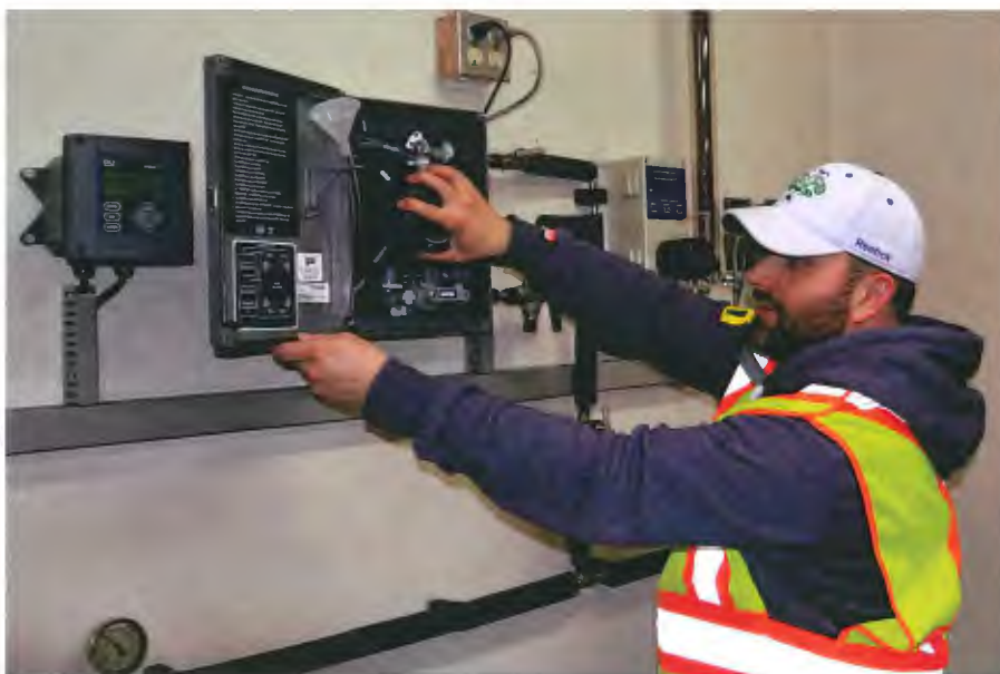
Inside a PRV station
