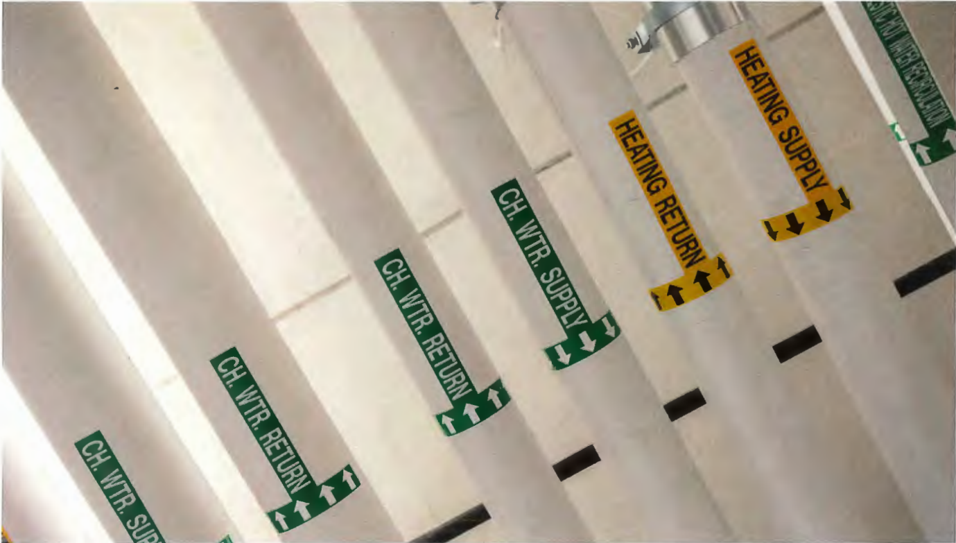
Interior supply and return piping located at the recently connected One Park.
