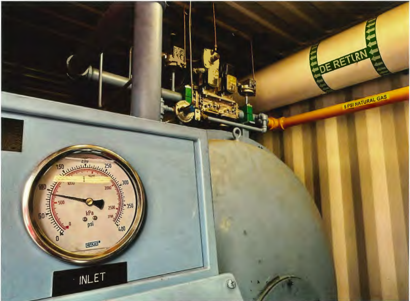
District energy infrastructure
