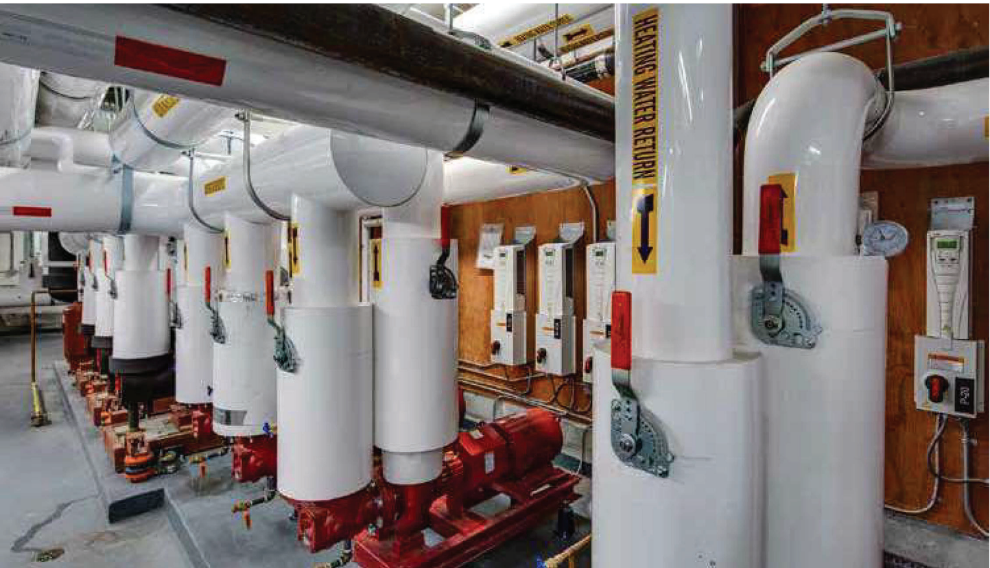
Mechanical infrastructure located in the CCDEUs first connected building: The Paramount.
