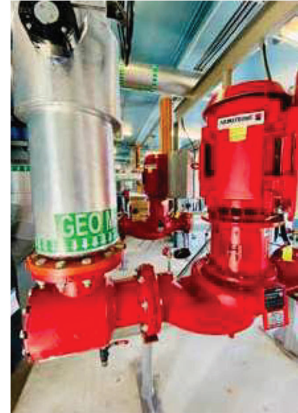
District energy piping inside the ADEU plant.
