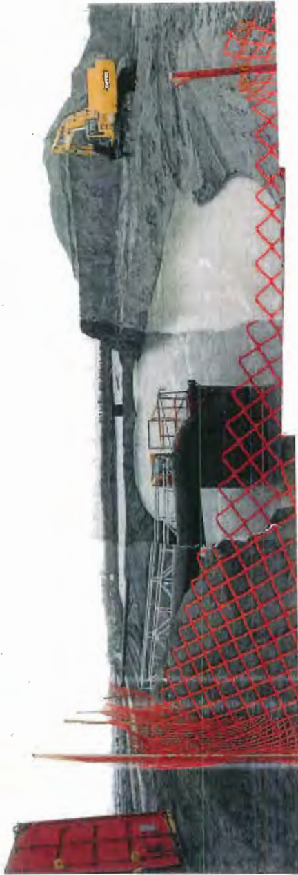
Pan view of dredge drainage water sump and pumping return to River
