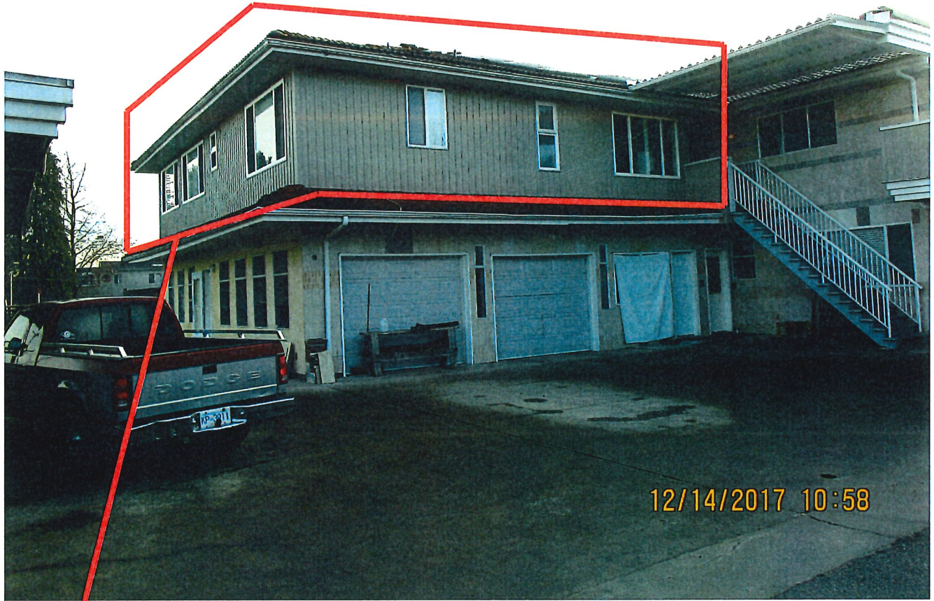
Second floor addition that contains two unauthorized suites
