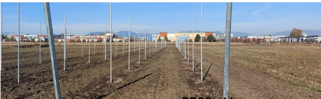
Galvanized posts installed in November 2022 to support a high density fruit tree orchard.
