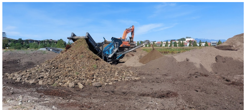
Equipment working at the site to screen the imported material prior to spreading across the site to ensure optimal quality. Sept. 2024
