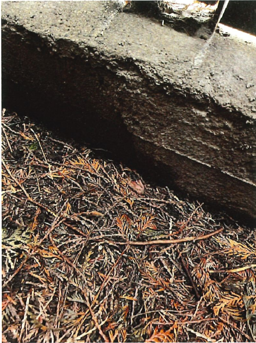
Phot 3 Cracks on CIP Concrete Retaining Wall
