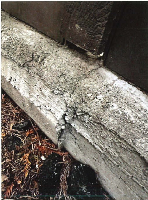
Photo 5 Cracks on CIP Concrete Retaining Wall
