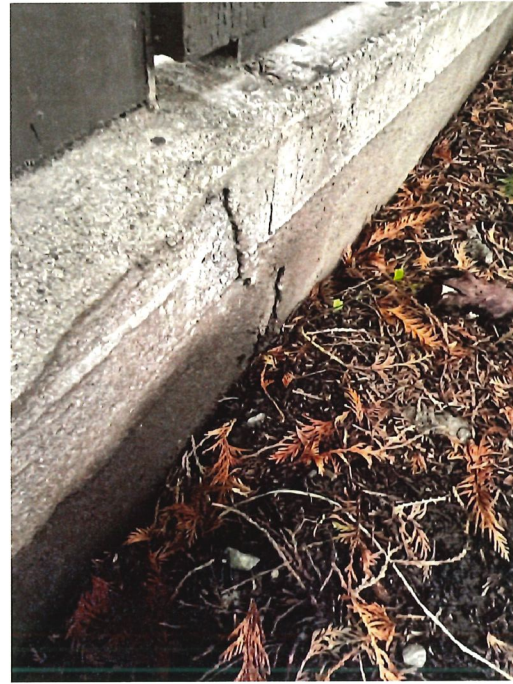
Photo 6 Cracks on CIP Concrete Retaining Wall
