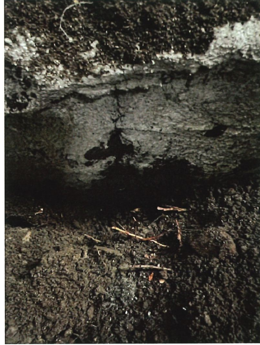
Phot 4 Cracks on CIP Concrete Retaining Wall
