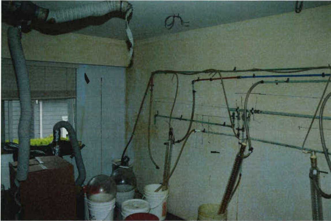
Image 6: production apparatus located in downstairs room. Heavy chemical staining on walls
