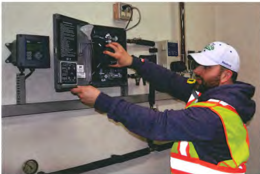
Inside a PRV station
