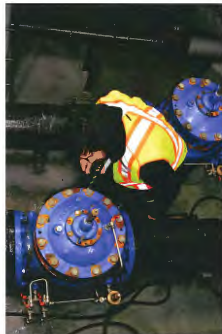
Inside a PRV station
