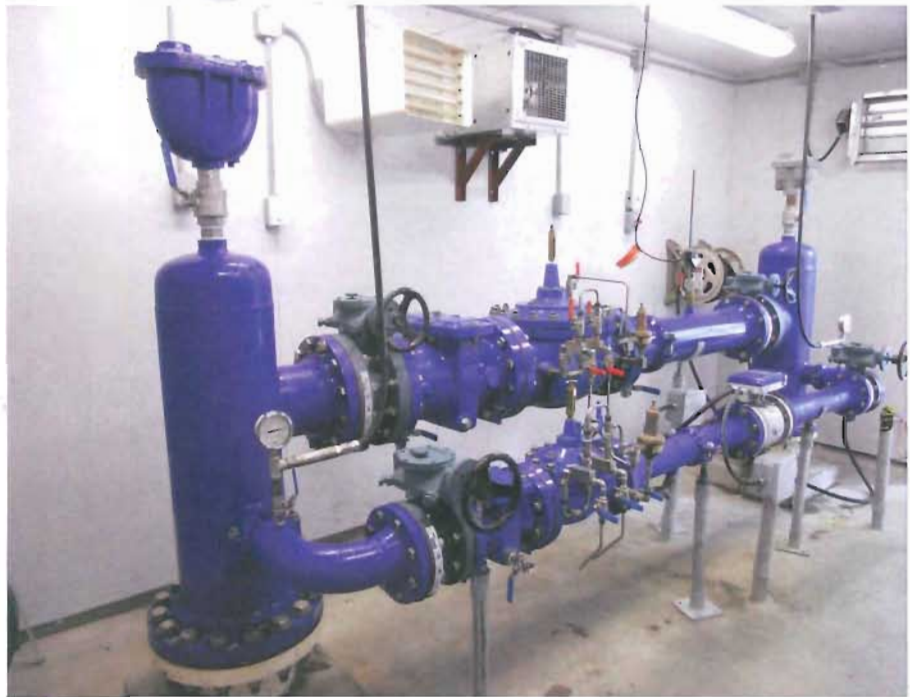
Nelson Road PRV Station
