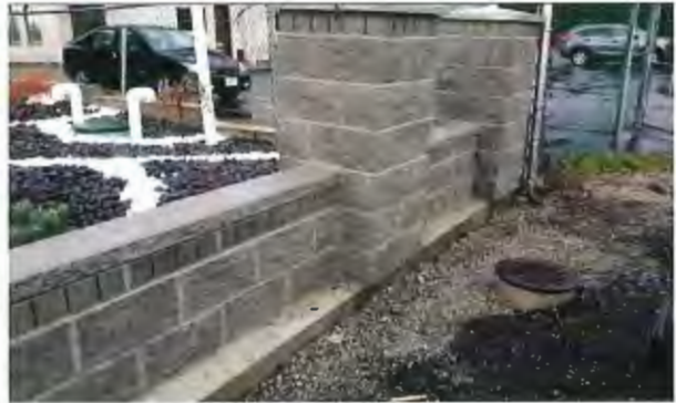
January 24, 2020 – Rim of inspection chamber located above surrounding ground elevation
