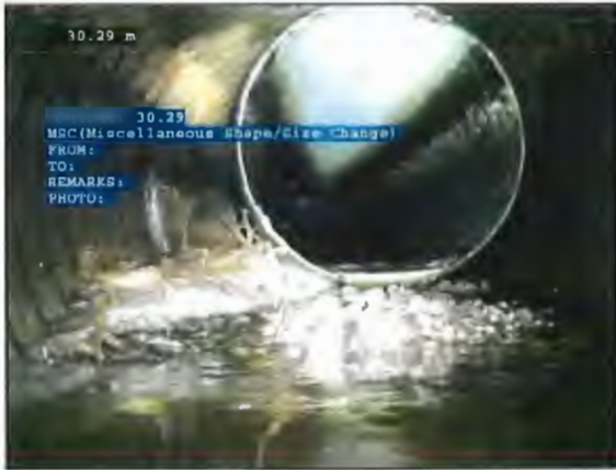
March 18, 2020 – CCTV unable to inspect unauthorized crossing due to missing manhole
