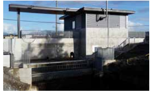
Bath Slough drainage pump station
