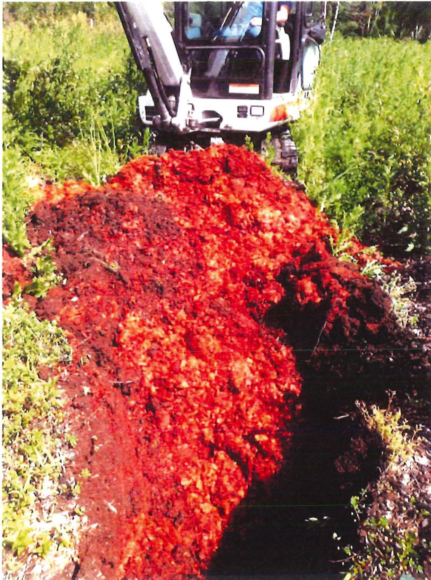
Figure 6: Buried Wood waste
