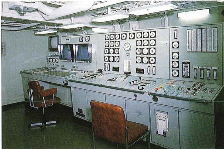
Engine control room
