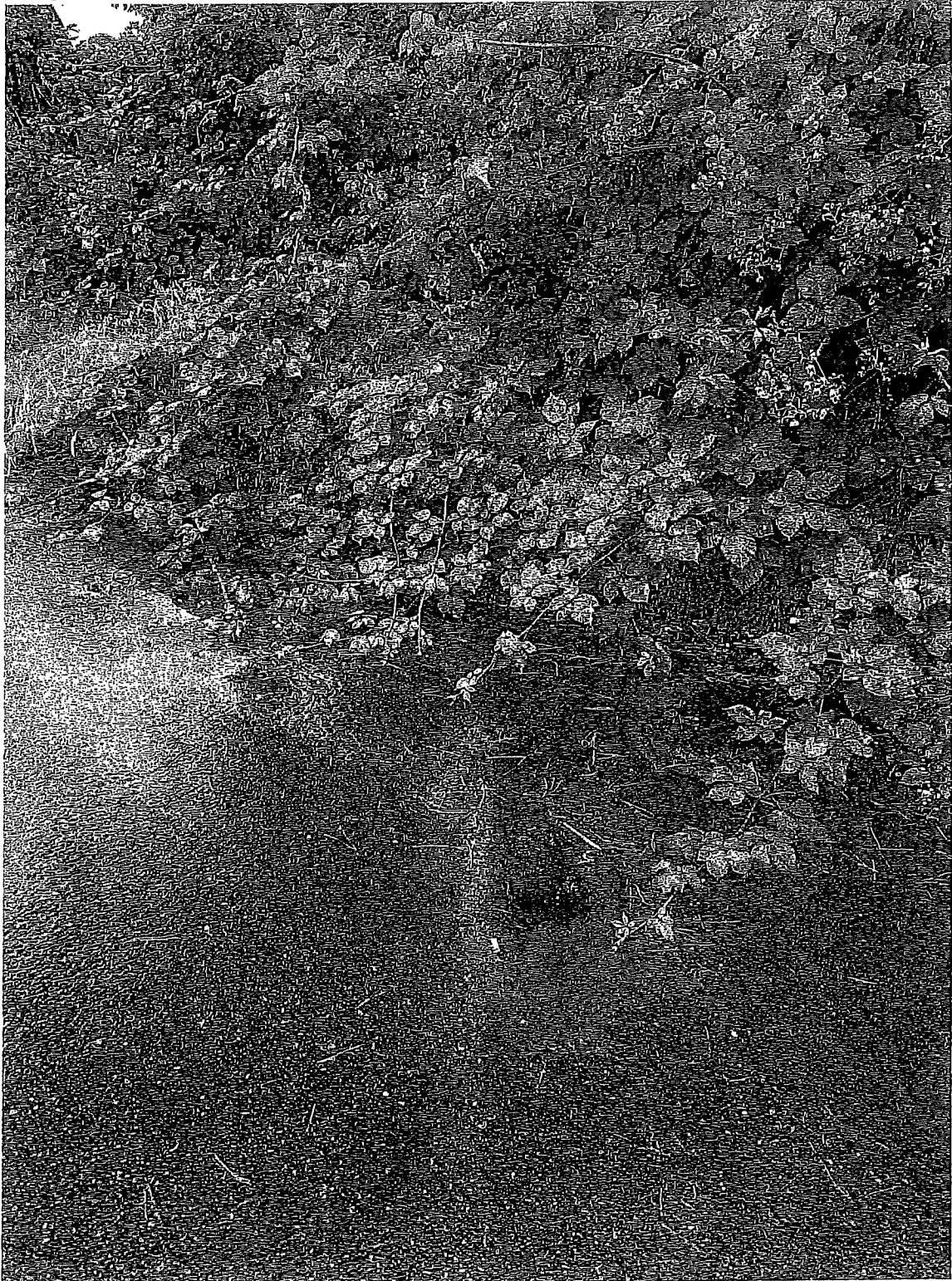
Overgrown bushes and brambles clogging a ditch facing Cook Crescent at a rental house.
