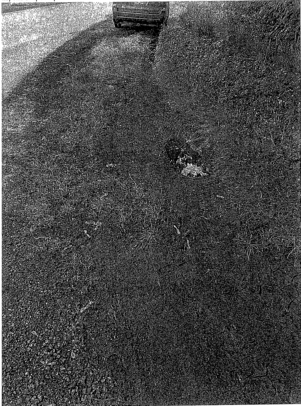
1b) The deep mudpit on the boulevard of one of the rental houses owned by Harry, on Cook Crescent.
