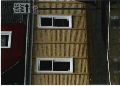
Example of white window opening trim and vertical trim matching siding colour.
