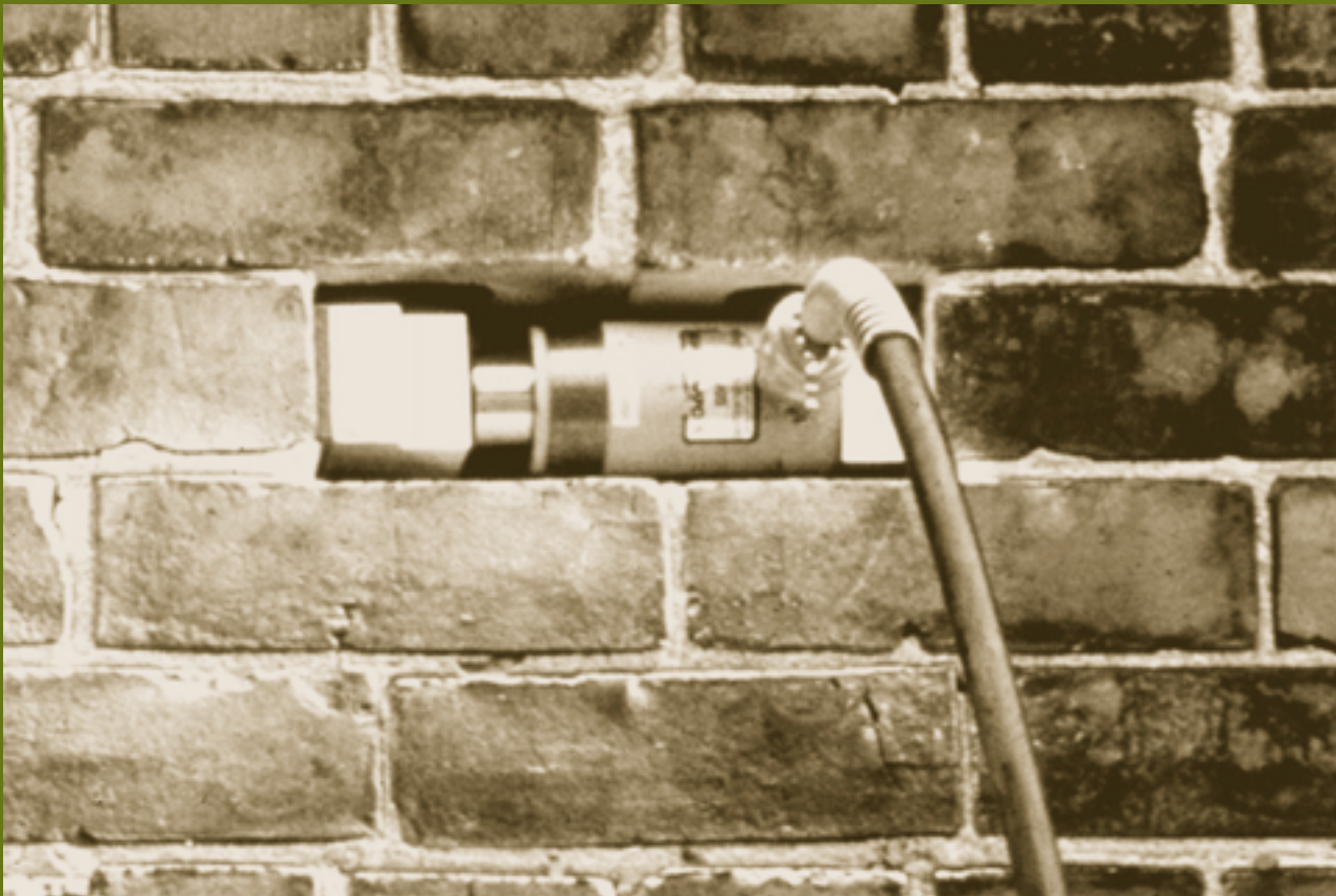
Minimally destructive testing techniques should be used to determine the strength of materials. For example, this in-place “push test” uses a calibrated hydraulic ram and a pressure gauge to measure the actual shear strength of a traditional brick wall, and thus its seismic resistance. A single brick beside the brick being tested is removed to accommodate the hydraulic ram (and is replaced in the wall after completion of the test).
