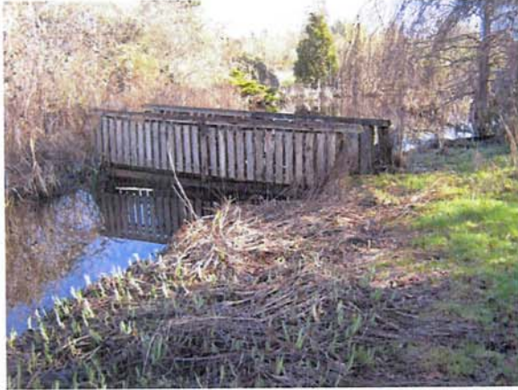
Wooden bridge – The decking and some of the structure needs to be replaced. Recommendation is to remove and replace.
