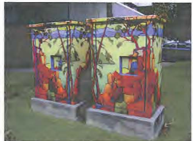
City Hall electrical kiosks Art Wraps, 2009
