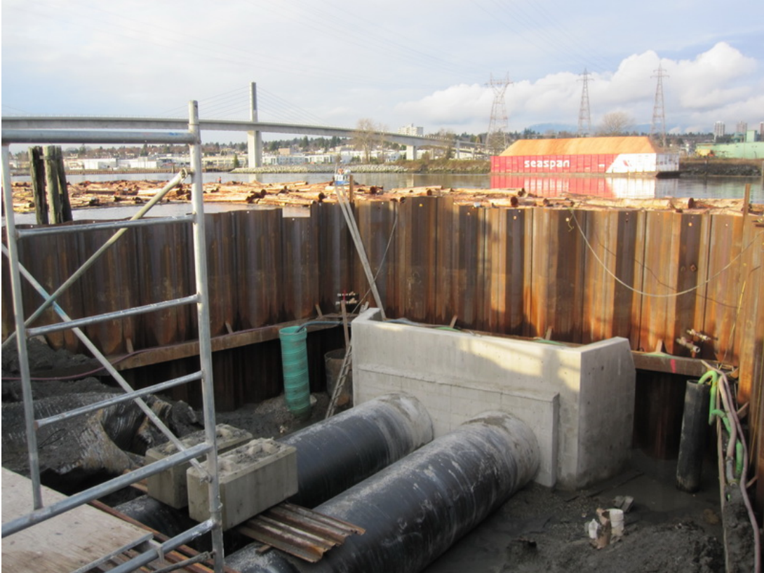
Gravity Discharge Pipes and Headwall
