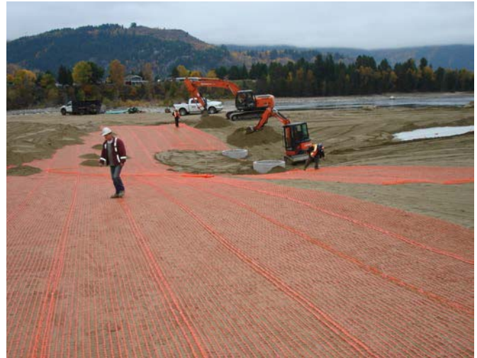
EXAMPLE: Indicator mesh installed on top of second sand cushion over liner. Additional sand cover installed over mesh.
