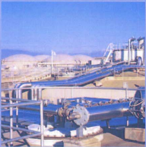
Annacis Island wastewater treatment plant provides treatment for over 1,000,000 people.
