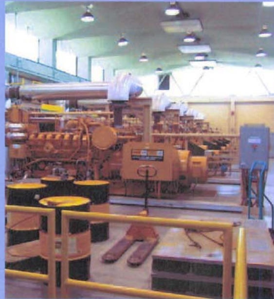
Biogas produced from wastewater supplies heat and power to the Iona Island wastewater treatment plant.
