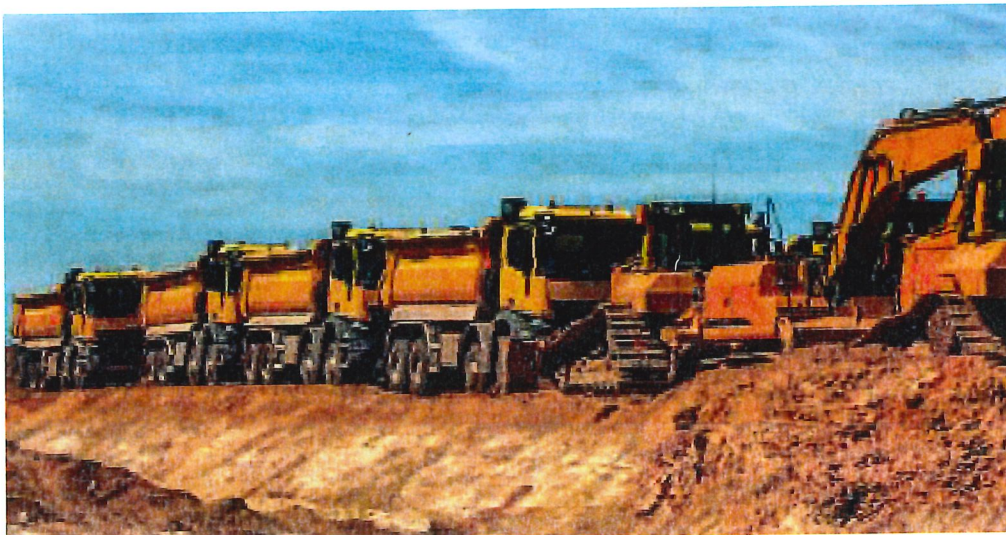
The Iona barge berth will replace approximately 500 dump trucks a day., That many trucks is the equivalent of lining up the trucks the length of the Grouse Grind.
