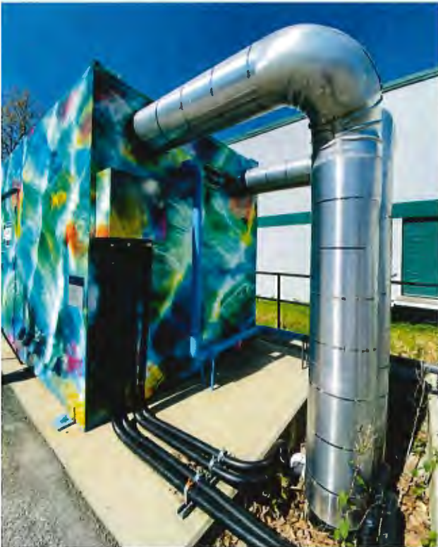
Oval Village District Energy Utility
