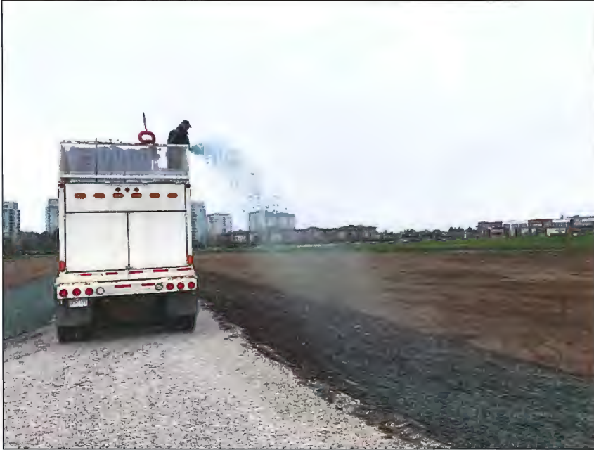
Above: Hydroseeding equipment applying native grass seed mixture to exposed soil slopes along farm access road.
