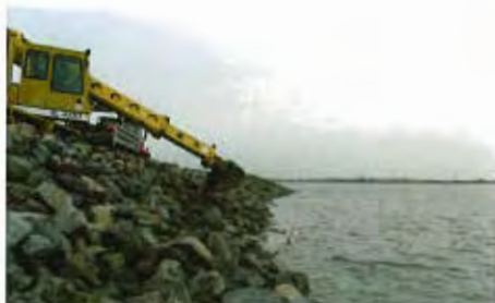
City crews continually maintain and upgrade the City's diking infrastructure. The Dike Master Plans Phases 1 to 5, anticipated for completion in 2019, specify upgrade requirements for Richmond's dikes according to current climate change science.
