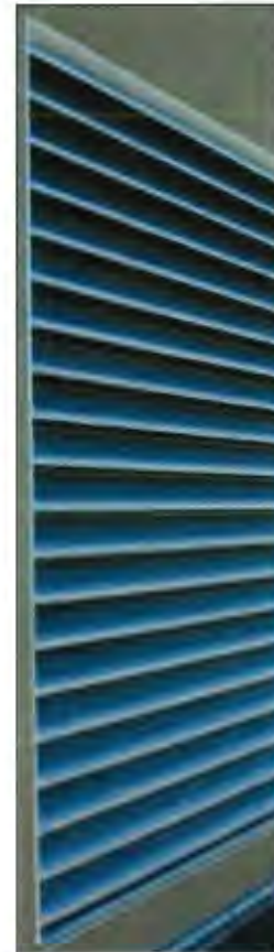
REFERENCE PICTURE MECHANICAL EXHAUST LOUVERS BEHIND ARCHITECTURAL SCREEN
