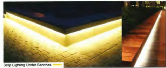
Strip Lighting Under Benches
