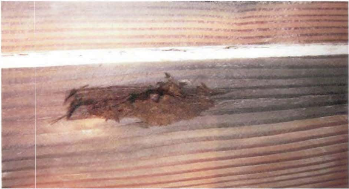
Photo #7 Detail of corroded fastener with adjacent deteriorated wood planking
