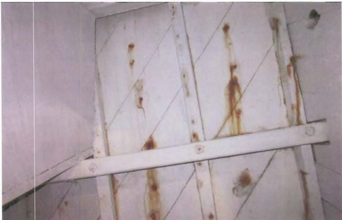
Photo #10 Detail of corroded fasteners inner planking
