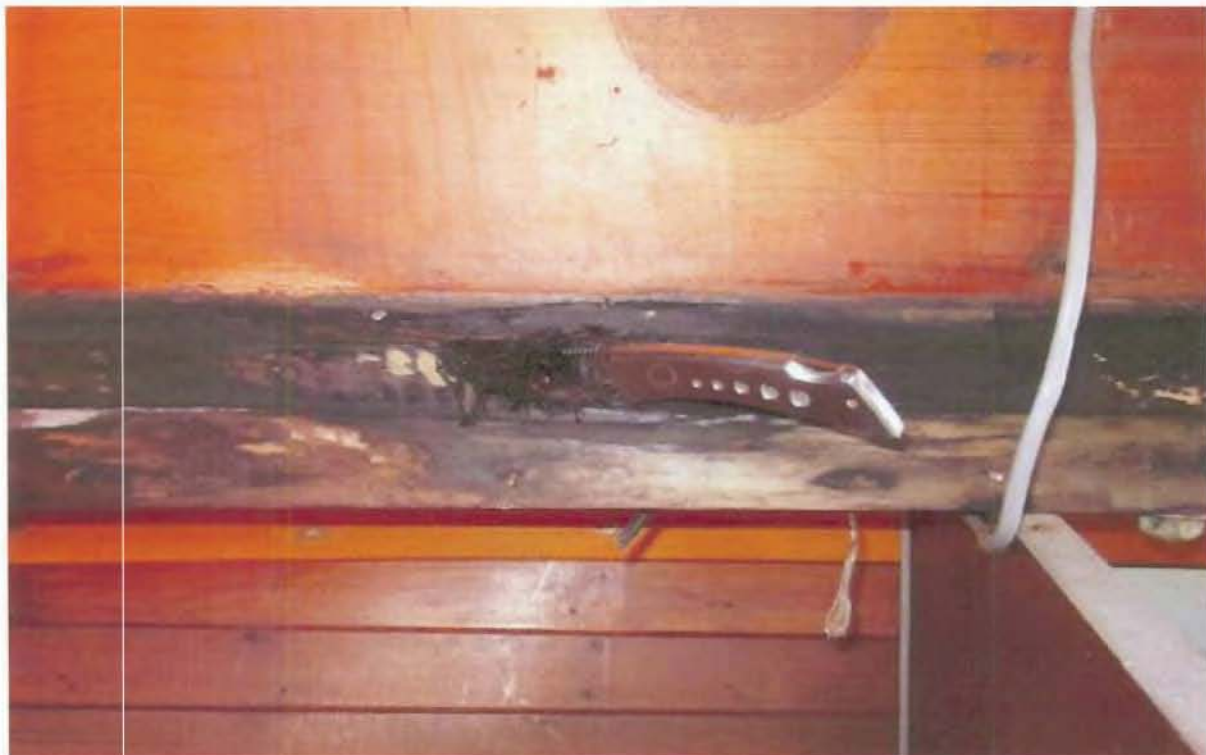
Photo #2 deterioration of side deck over carlin plank
