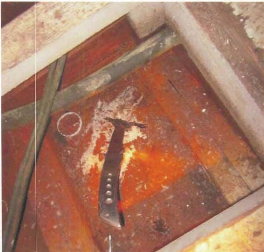
Photo #8 Deterioration of inner planking
