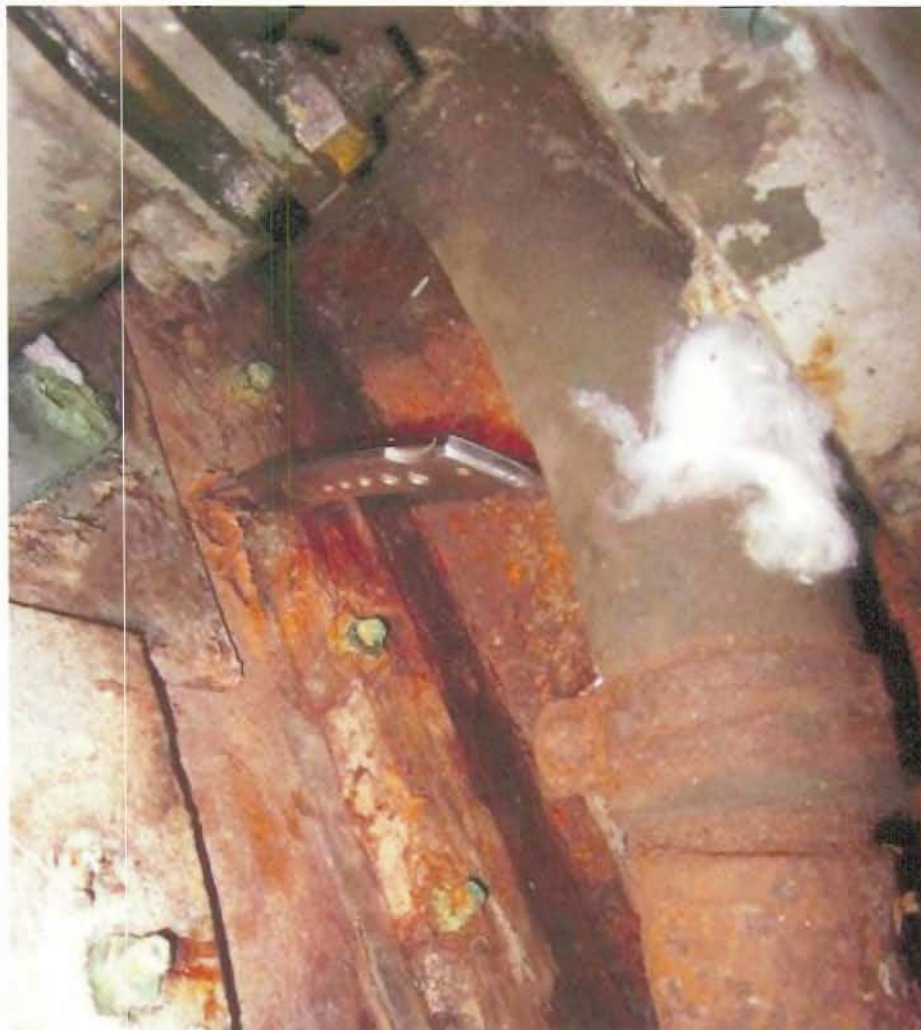
Photo #4 Deterioration of bulkhead under engine stern tube
