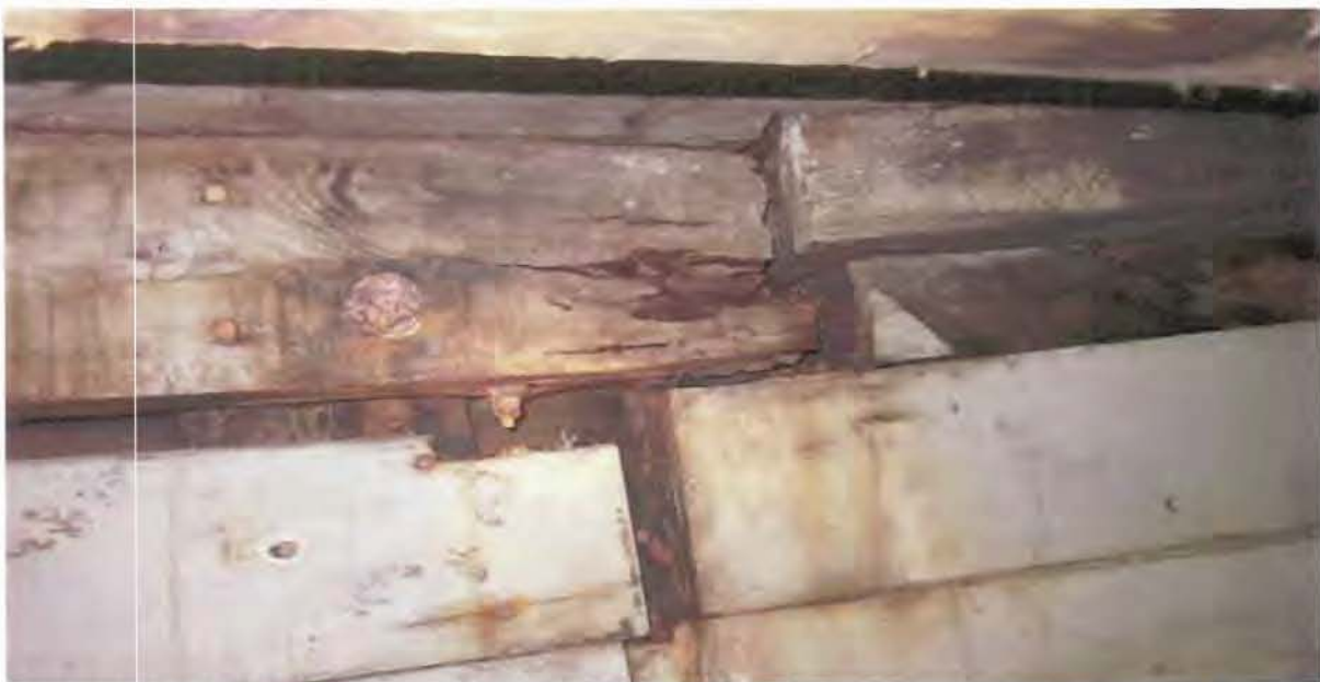
Photo #1 Detail of deterioration in hull framing stern section
