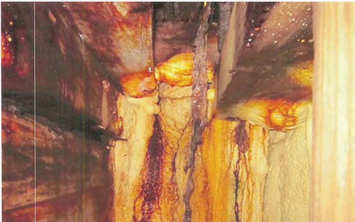
Photo #3 Detail of deterioration at fish hold foam/hull connection
