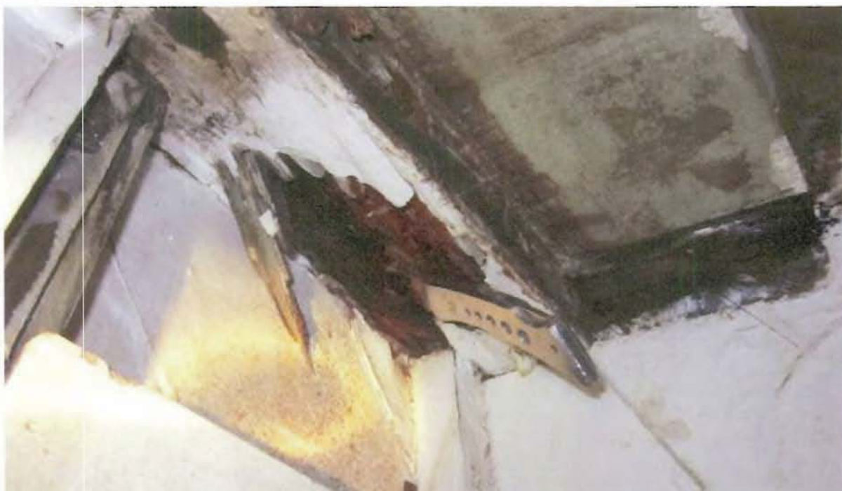
Photo #5 Deterioration of sheer clamp forward cabin
