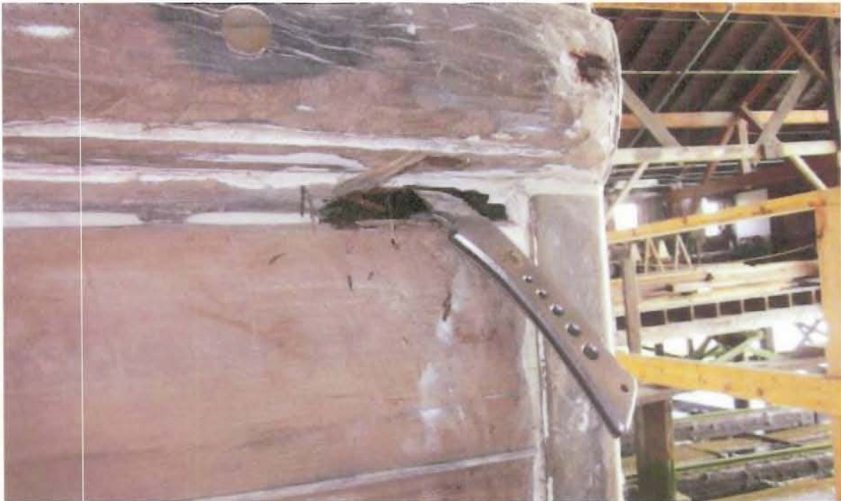
Photo #9 Deterioration of transom exterior planking starboard corner
