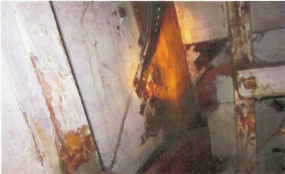
Photo #2 Deterioration of inner transom structure
