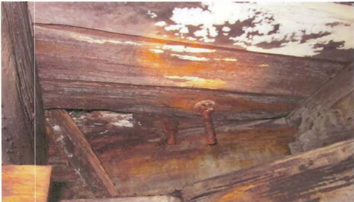
Photo #2 Detail of deterioration under aft deck and transom/hull connection
