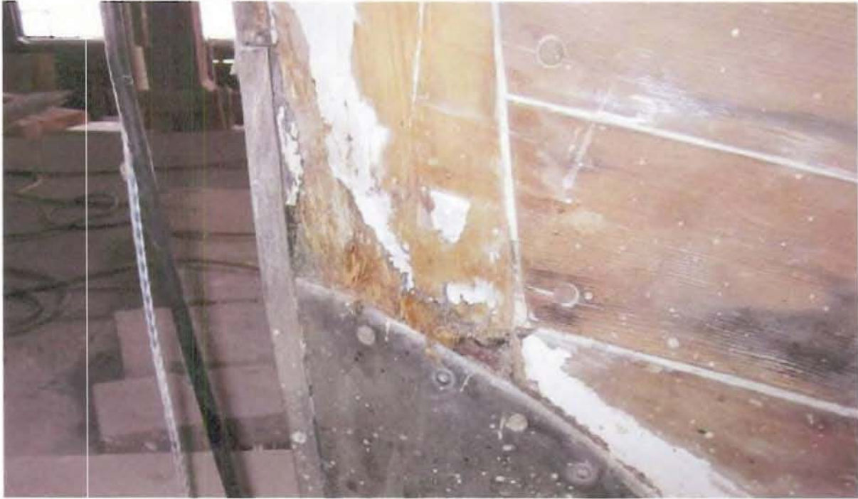
Photo #1 Damage of exterior stem structure
